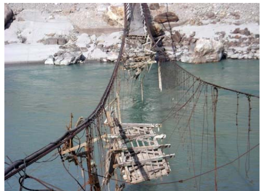
Flood destroyed foot bridge - Indus River, Gilgit Baltistan
