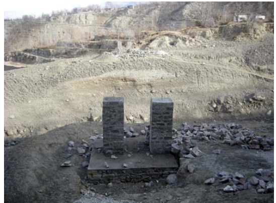
Foundations of a foot bridge are laid on a trekking route in Gilgit Baltistan
